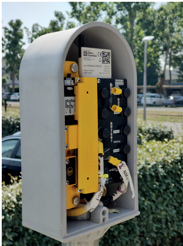
Figure 4 Kairos installed in the field
